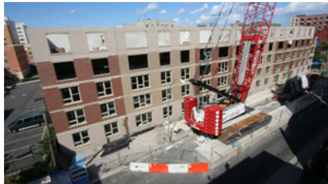
The complex is being built on East 156th Street between Melrose and Elton avenues in the South Bronx. The one-, two- and three-bedroom units are for families with incomes below 60% of New York City's adjusted median income.
